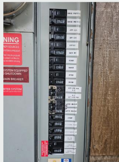
Figure 8. Circuit Breakers Close Up
