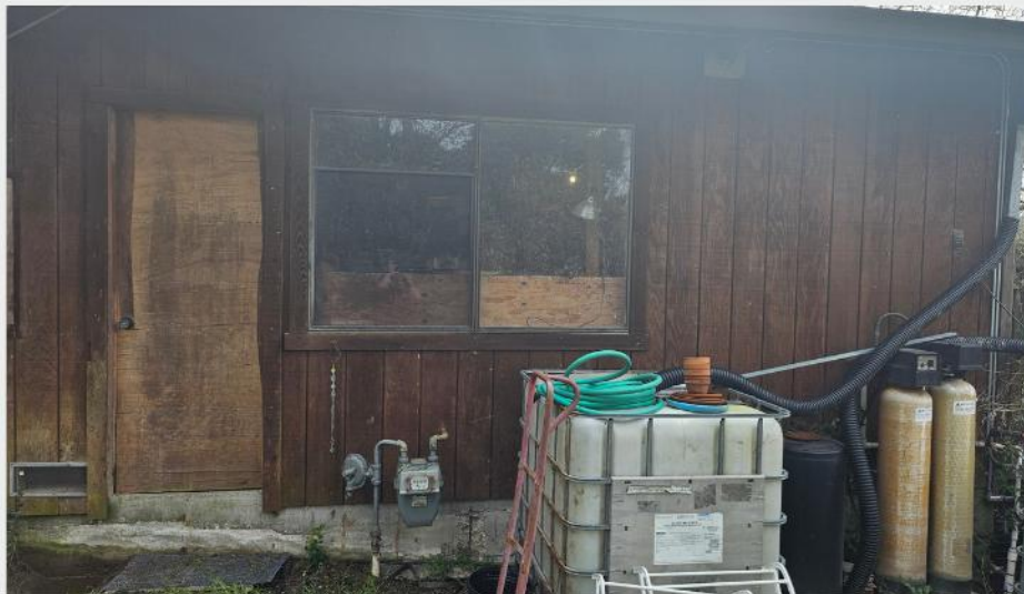
Figure 11. Gas Meter/Water collection tank.
