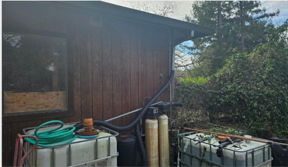
Figure 9. Water Collection System
